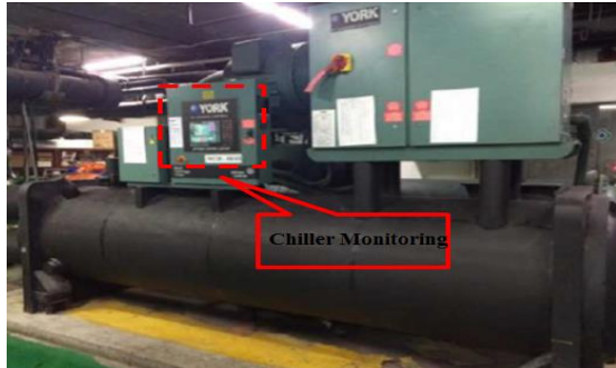
Fig. 2 Chiller room of TM 1
